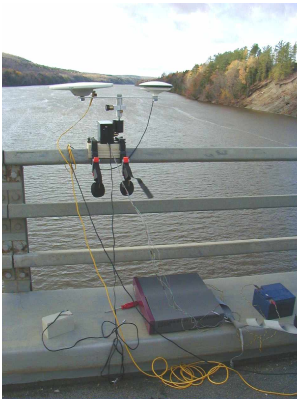
FIGURE 6 -- GPS antennas, reflector target and accelerometer housed together on the guardrail of middle center span of Hawkshaw Bridge
